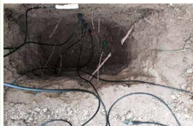
Farmers, young researchers, graduate students, and extension staff installing equipments as part of the series on-farm trials carried by ICBA and its partners for better on-farm water management.
